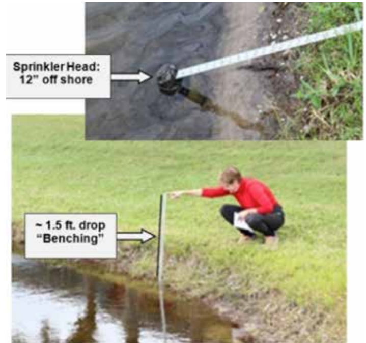
Shoreline erosion at Rivendell Ponds is real and visible. LMZs & plantings will help control pond shoreline damage.
